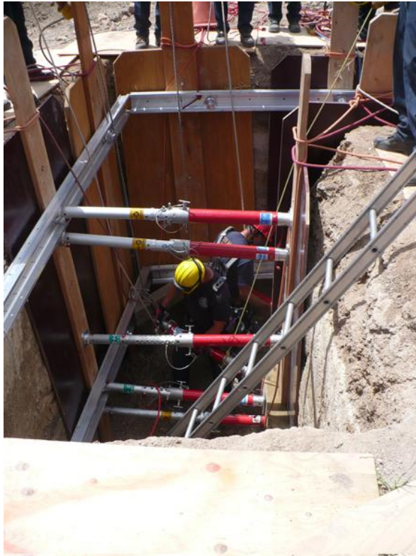
Figure 9-19 Create a safe zone in the uncollapsed portion of the trench by using appropriate protective systems
