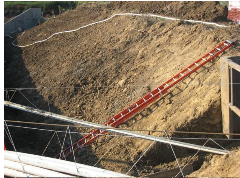
Figure 9-20 Secure all utilities, pipe, and any other obstruction in the trench not already secured due to inaccessibility issues
